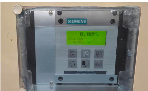
Figure 6-7: Goal 6 Electromagnetic Flow Meters Used for Monitoring and Collecting Water Consumption Data
